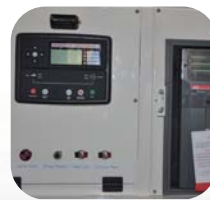
Control Panel & MCB
